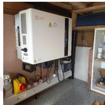
Figure 15: PV Battery storage installed thanks to the CIG.
